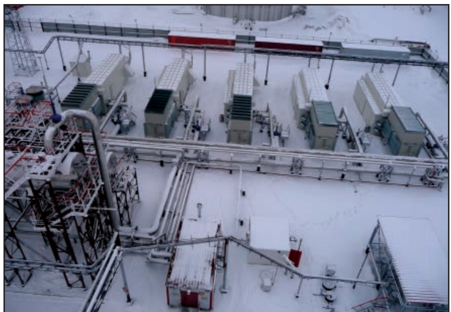
The West Siberia station was constructed in 2008. Gas delivery pressure is 232 psi (16 bar). Gas flow for each of the five Enerproject-supplied units is 247,202 cfh (7000 Nm 3 /hr).
